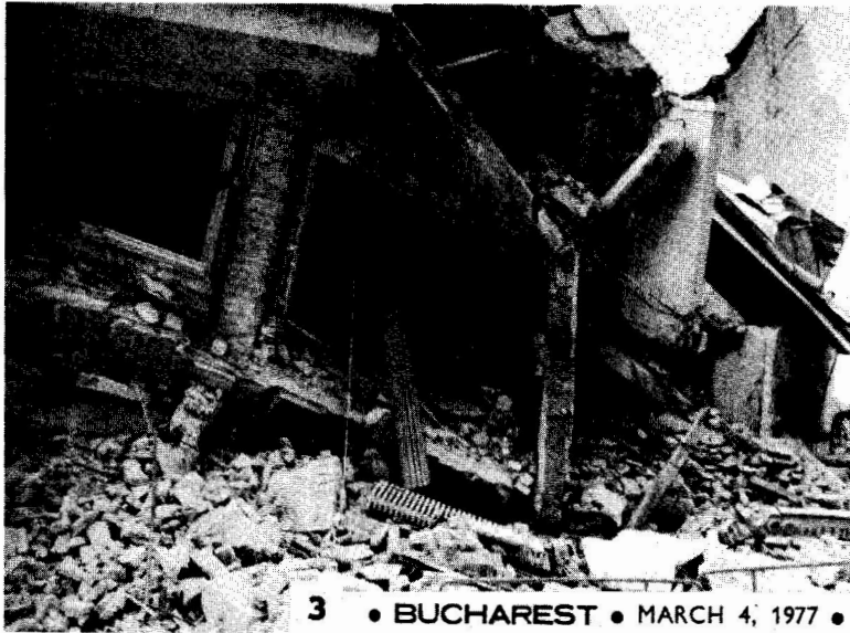
Collapsed block of flats with soft ground floor (erected before 1940)
